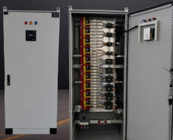
Power Factor Correction Panels
